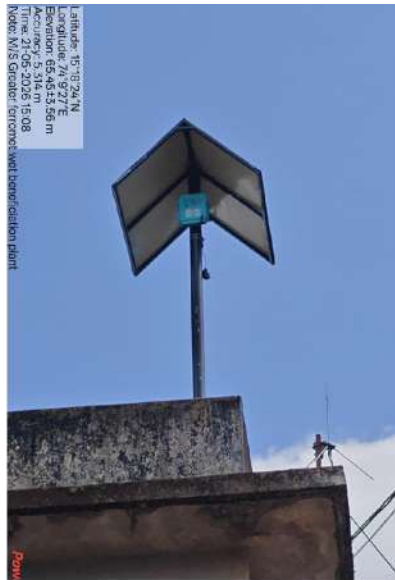
Greater Ferromet Plant
